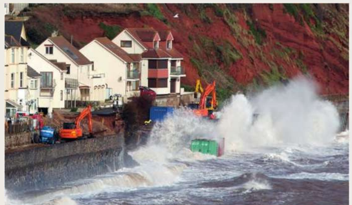
Figure 3.1: Waves are very powerful during storm conditions, such as here at Dawlish in Devon in February 2014. How does the destruction shown in the photograph demonstrate the power of the sea and the rate of possible change?
