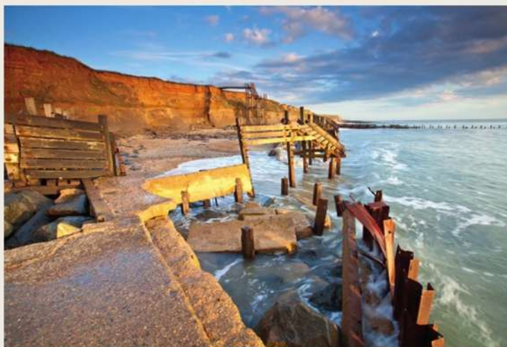
Figure 3.33: Failed defences and coastal erosion at Happisburgh, Norfolk
